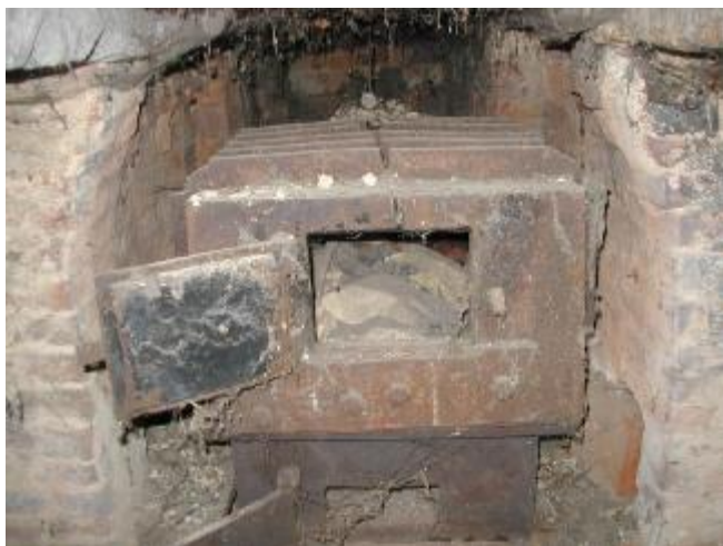
Figure 8 – North door fire box
